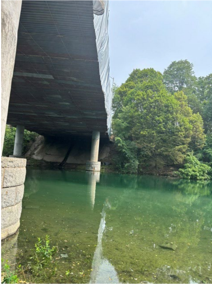
Class A paint containment system
